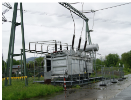
(c) Three-phase transformer (source: Wikimedia Commons , Asurnipal, CC BY-SA 4.0)
