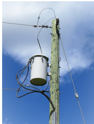
Fig. 3.1: Transformer integrated at a utility pole (source: pxhere.com , public domain)
