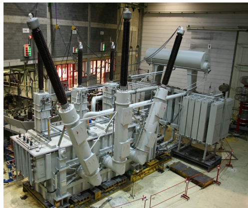
Fig. 3.27: 750 MVA, 380 kV / 230 kV three-phase autotransformer (source: Wikimedia Commons , P. Mertens, CC BY-SA 3.0)
