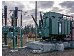
(b) Single-phase transformer (source: Wikimedia Commons , Georg, CC BY-SA 4.0)
