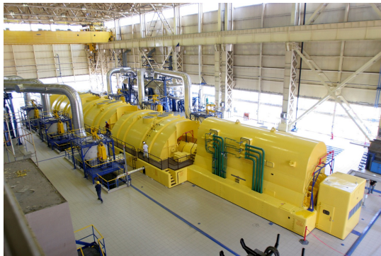
(a) 650 MVA turbogenerator from Cernavodă nuclear power plant (source: Wikimedia Commons , R. Lavinia, CC BY-SA 4.0)
